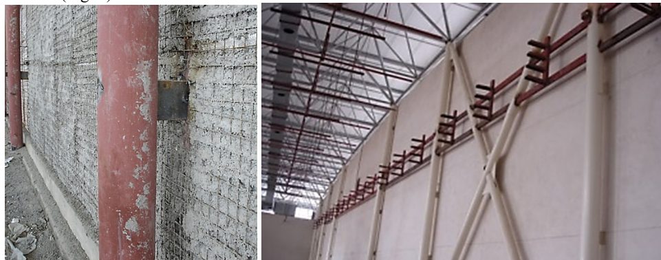
Fig. 6. Sudden change in the slenderness (left) and punching the columns and braces in order to pass the utility pipes (right)
