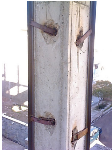
Fig. 4. Unauthorized concrete tampering and welding some architectural parts to bars
